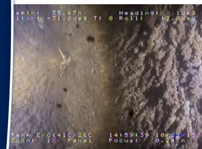
Conduit valve fault identified – 35 mtr depth
